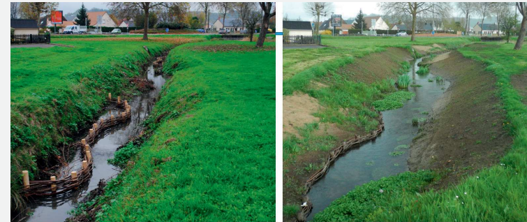
Ecological restoration of a watercourse in the commune of La Flèche, France
